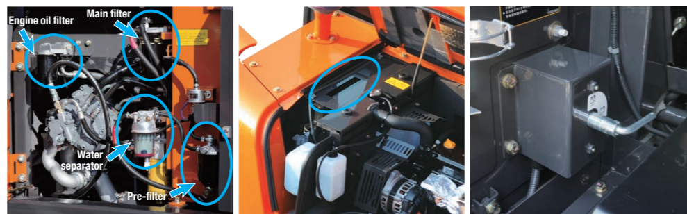
Grouped remote filters and inspection points
